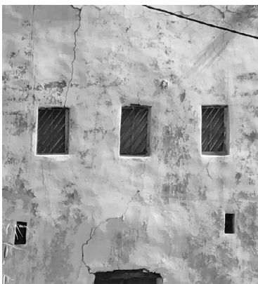
Punched / ventilation openings
